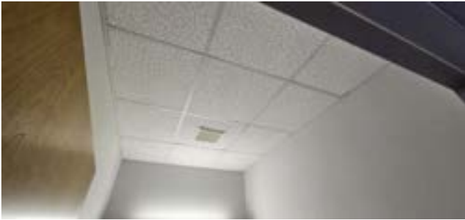
5.6 Bath Ventilation: Serviceable
