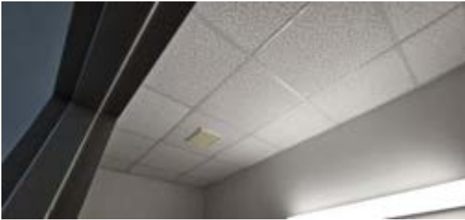
5.17 Bath Ventilation: Serviceable
