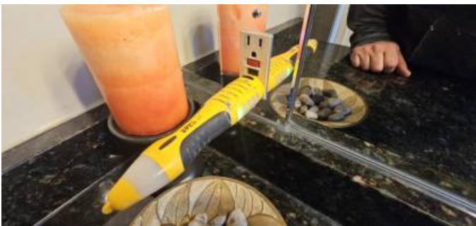
7.59 Switches/Outlets/Fixtures: A representative sampling of switches and outlets were tested. As a whole, outlets throughout the room are in serviceable condition.
